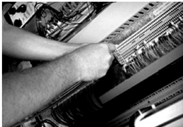
Panel being connected to a simulator for functional testing
